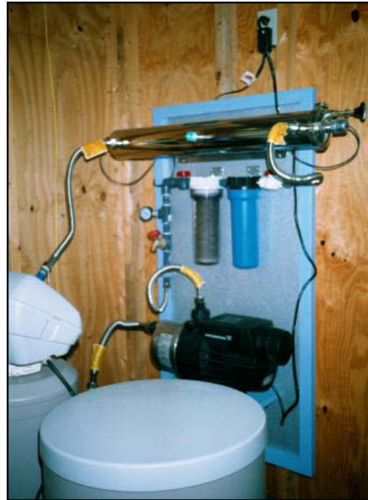
Figure 2-12. Typical treatment installation of an on-demand pump, 5-micron fiber filter, 3-micron activated charcoal filter, and an ultraviolet lamp (top).
